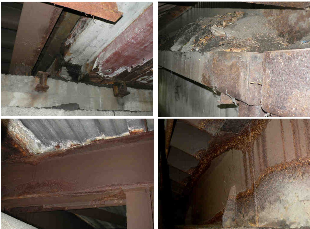
Figure 6: Effect of leaked precipitation with de-icing salt content
